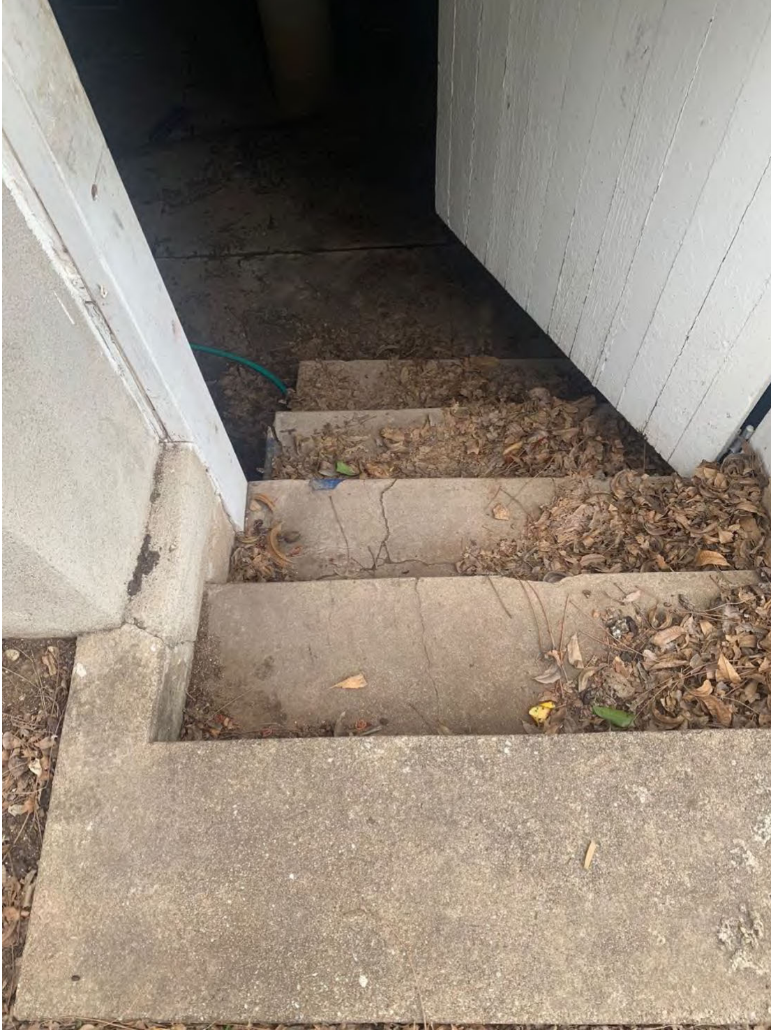
Photo 9 Stairs to crawlspace under back porch Camera facing north into space Photo by Tere O'Connell
