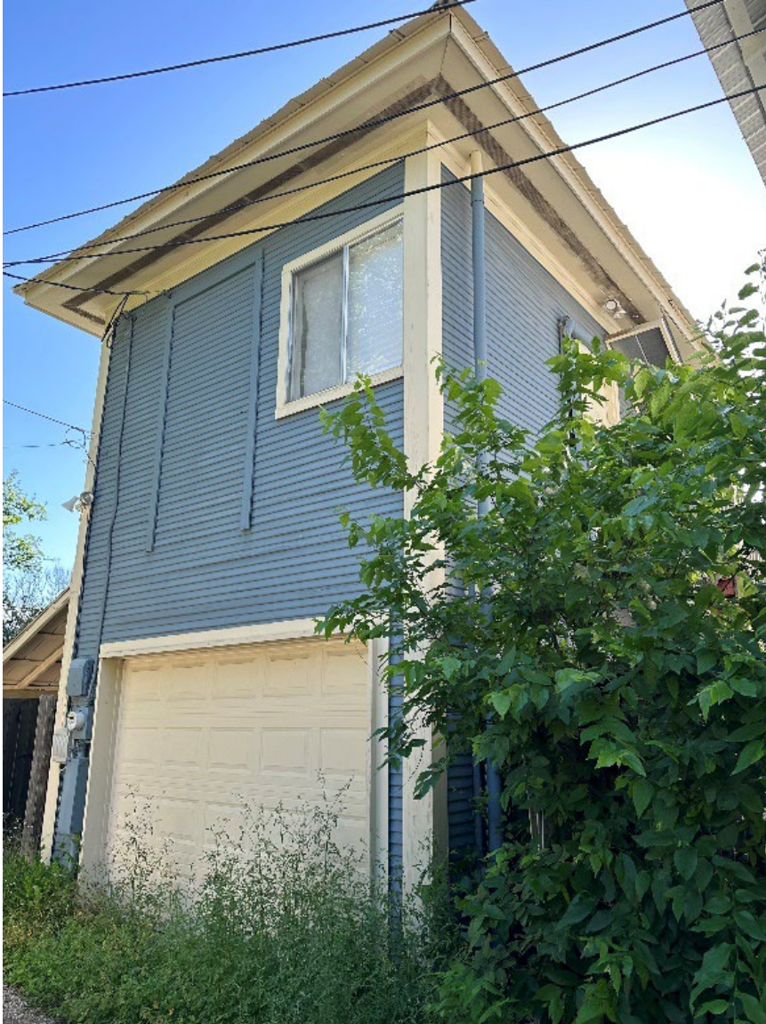
Photo 16. Oblique view of rear Garage, camera facing northeast, 4310 Avenue H. Photo by HHM, April 2024.
