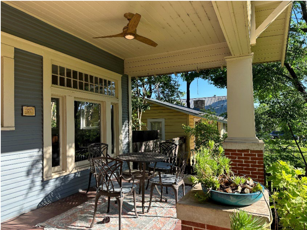
Photo 4. Detail of north end of primary façade, camera facing northwest, 4310 Avenue H. Photo by HHM, April 2024.
