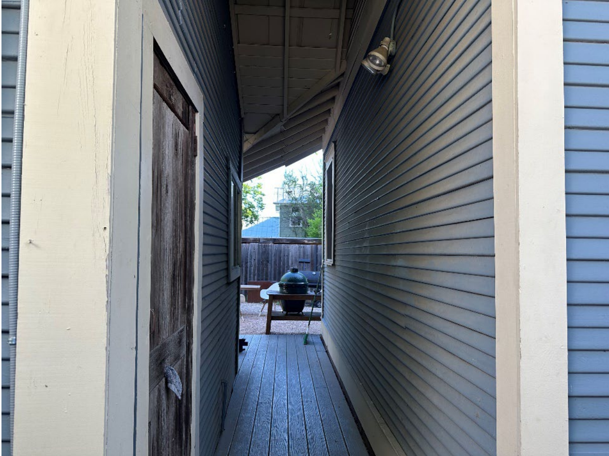
Photo 10. South façade view of outdoor hallway between main building and rear addition, camera facing north, 4310 Avenue H. Photo by HHM, April 2024.
