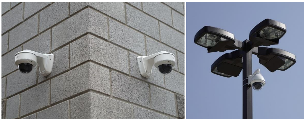
Figure 16. Examples of wall mounted (left) and light pole mounted (right) video surveillance cameras.
