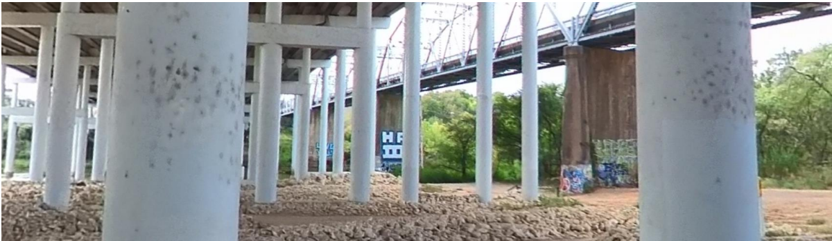
Picture C-39. Colorado River Wildlife Sanctuary - extensive graffiti covers the pedestrian bridge pillars
