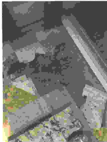
Asbestos Containing Floor Tile 1 st Floor Hallway 2% Chrysotile Floor Tile None Detected-Mastic
