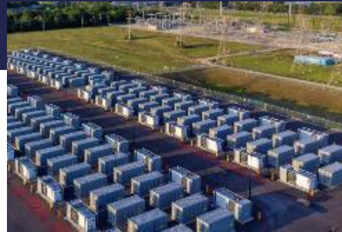
Utility-Scale Battery Project
